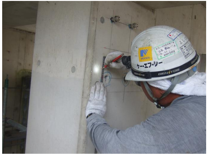
Upper: Chemical anchor M16 Lower: Marking for Deflective Anchor Bolt at a position where there is a re-bar.
