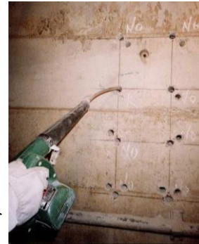
<Deflective Anchor Bolts are used at seven points out of eight points>
