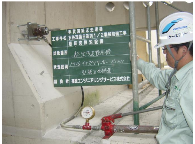
<No abnormality under 25 kN pull-out load>
